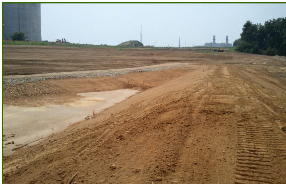
The construction is underway for a second solar power field at UGI.
